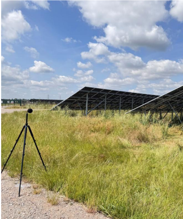
Figure 4: String inverter monitoring - daytime
