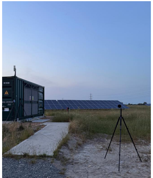
Figure 7: Transformer monitoring - twilight
