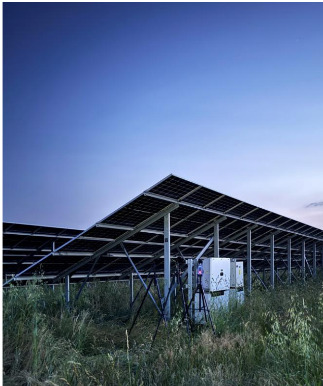
Figure 6: String inverter monitoring - twilight
