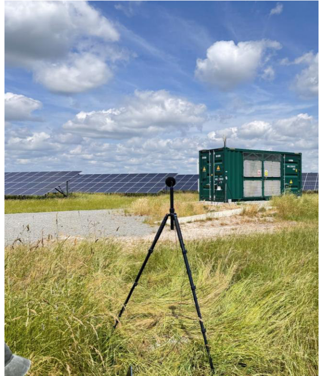
Figure 5: Transformer monitoring - daytime
